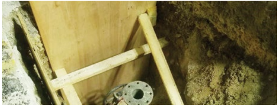
Figure 3: Installed entry port for the SmartBall was outside the special pad area of the light rail tracks
