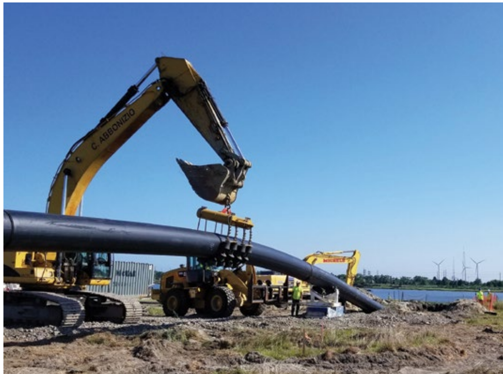
The 30-inch diameter HDPE PE 4710 pipe being pulled backward in the HDD process. (PHOTO COURTESY OF ACUA)
