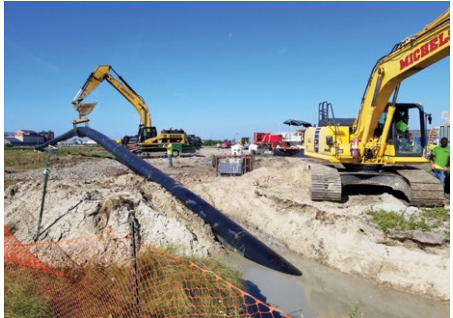
The 30-inch diameter HDPE PE 4710 pipe enters the HDD path to go under the Beach Thorofare waterway. (PHOTO COURTESY OF ACUA)
