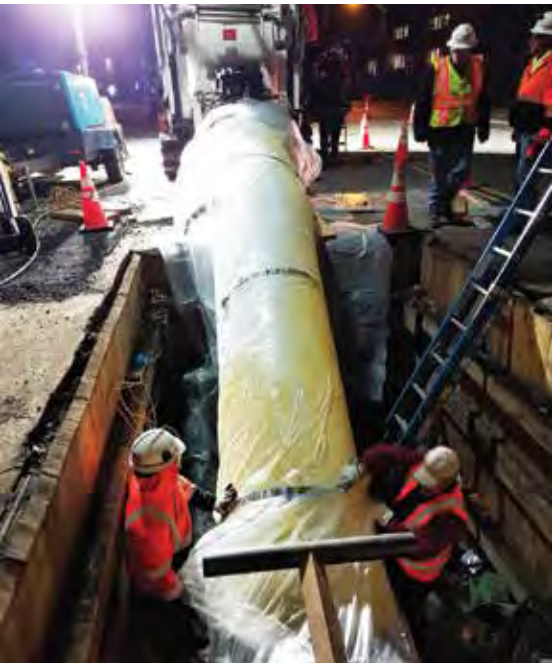
Starline® Cured in Place Liner coming off the drum guided as it enters the host pipe
