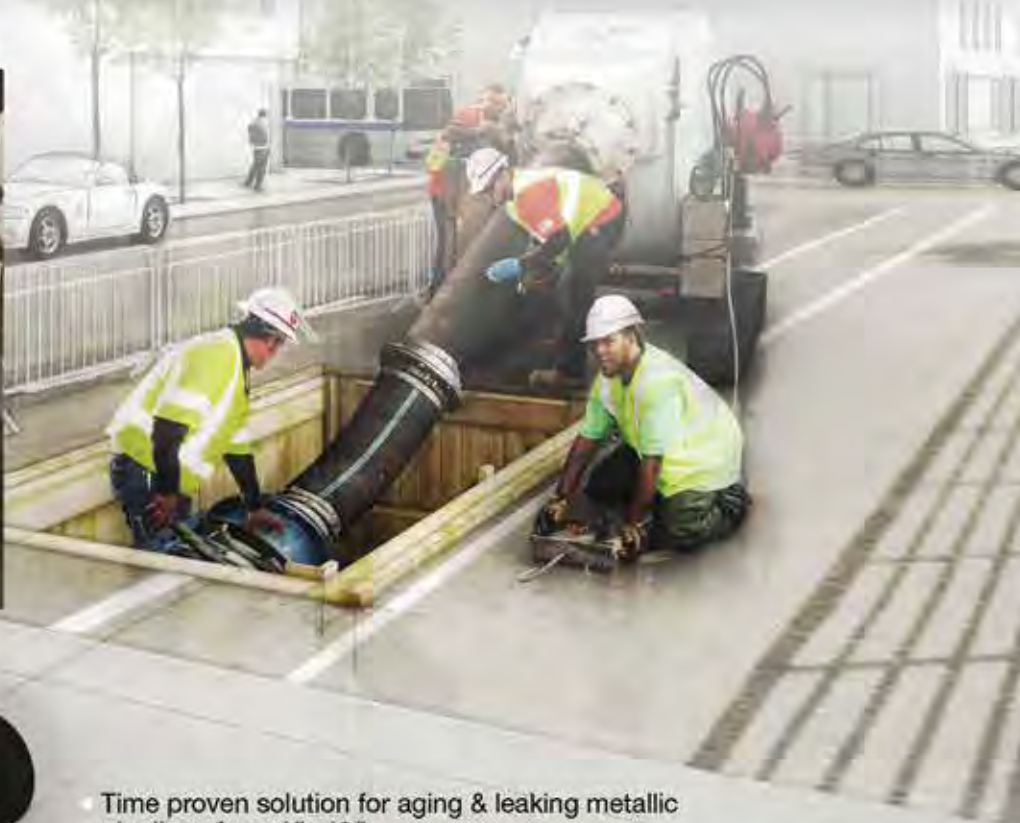
PPM / Starline holds the world record for the largest gas main ever lined. 36" Cast Iron Main, Seton Hall, NJ, November 2017
