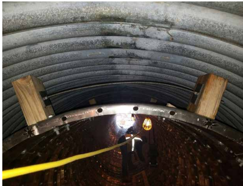
Blocking between Tunnel Liner Plate and host pipe ensured worker safety and provided uplift resistance during grouting
