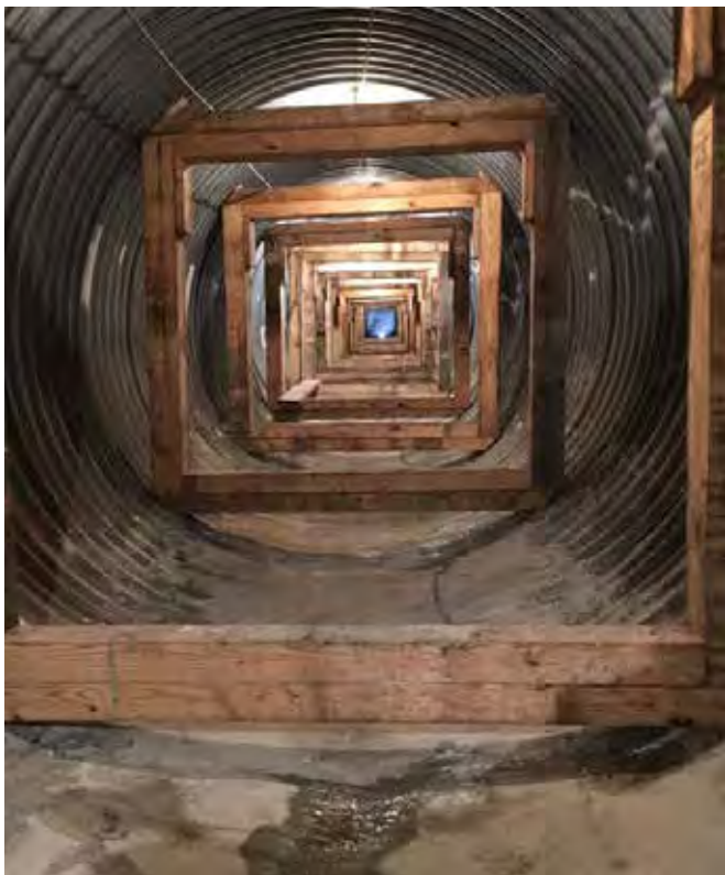
Host pipe stabilized with box beam frames to temporarily address structural concerns
