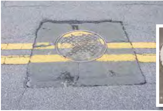
Often the concrete pad is damaged, cracked, and uneven
