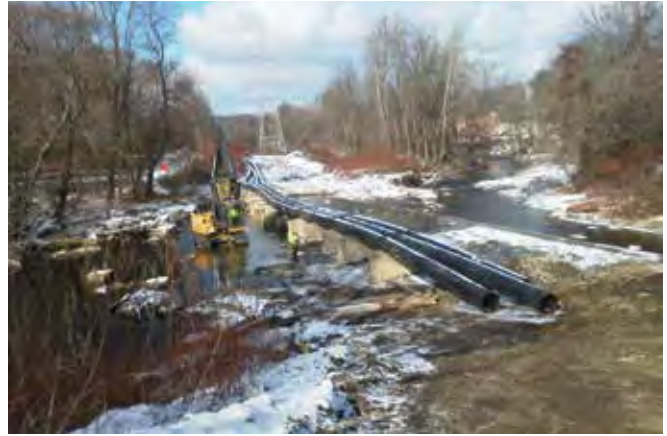
Figure 8 – Bypass Piping Crossing Ohio Canal near LCR
