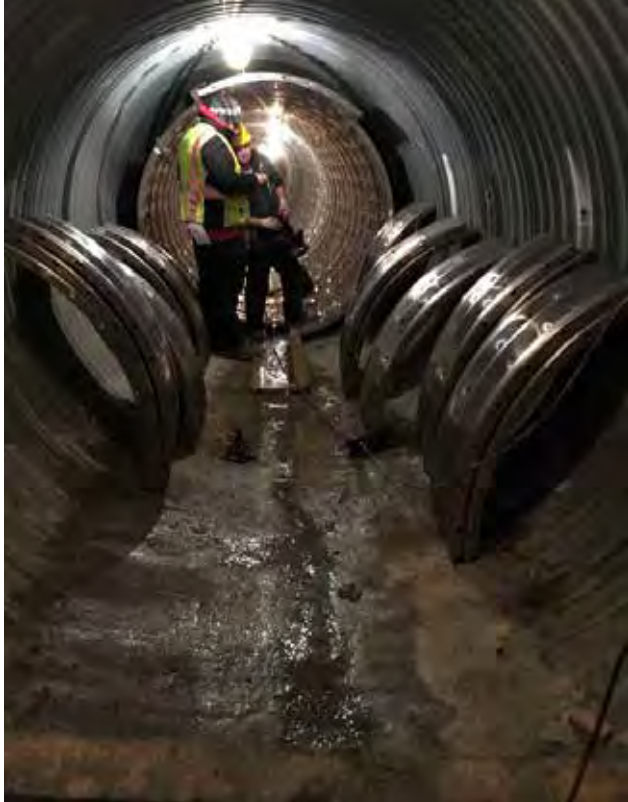
Individual sections were assembled inside the host pipe; 5 plates for each pipe ring
