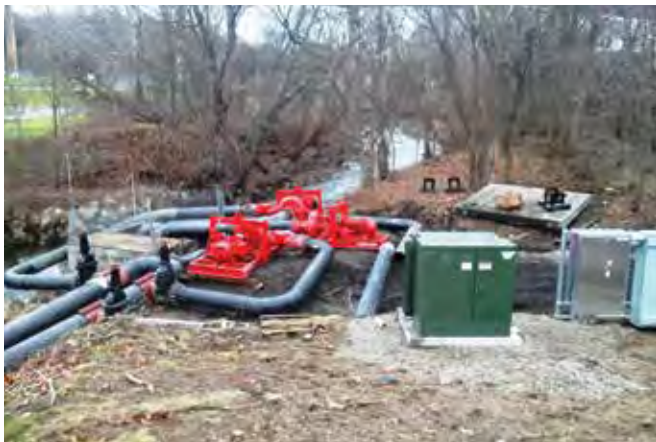
Figure 6 – Bypass Pump Setup
