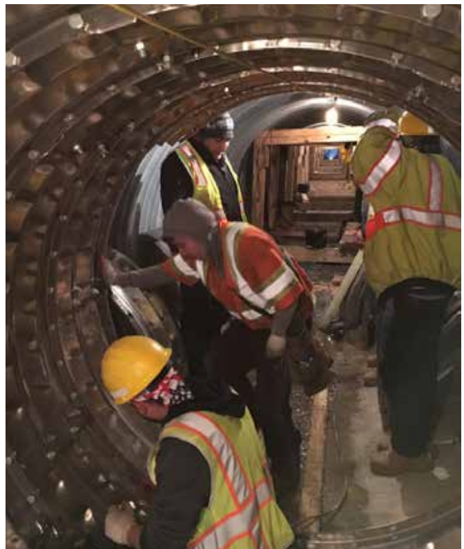
Tunnel Liner Plate provided a safe working environment as workers progressed through the length of the structure
