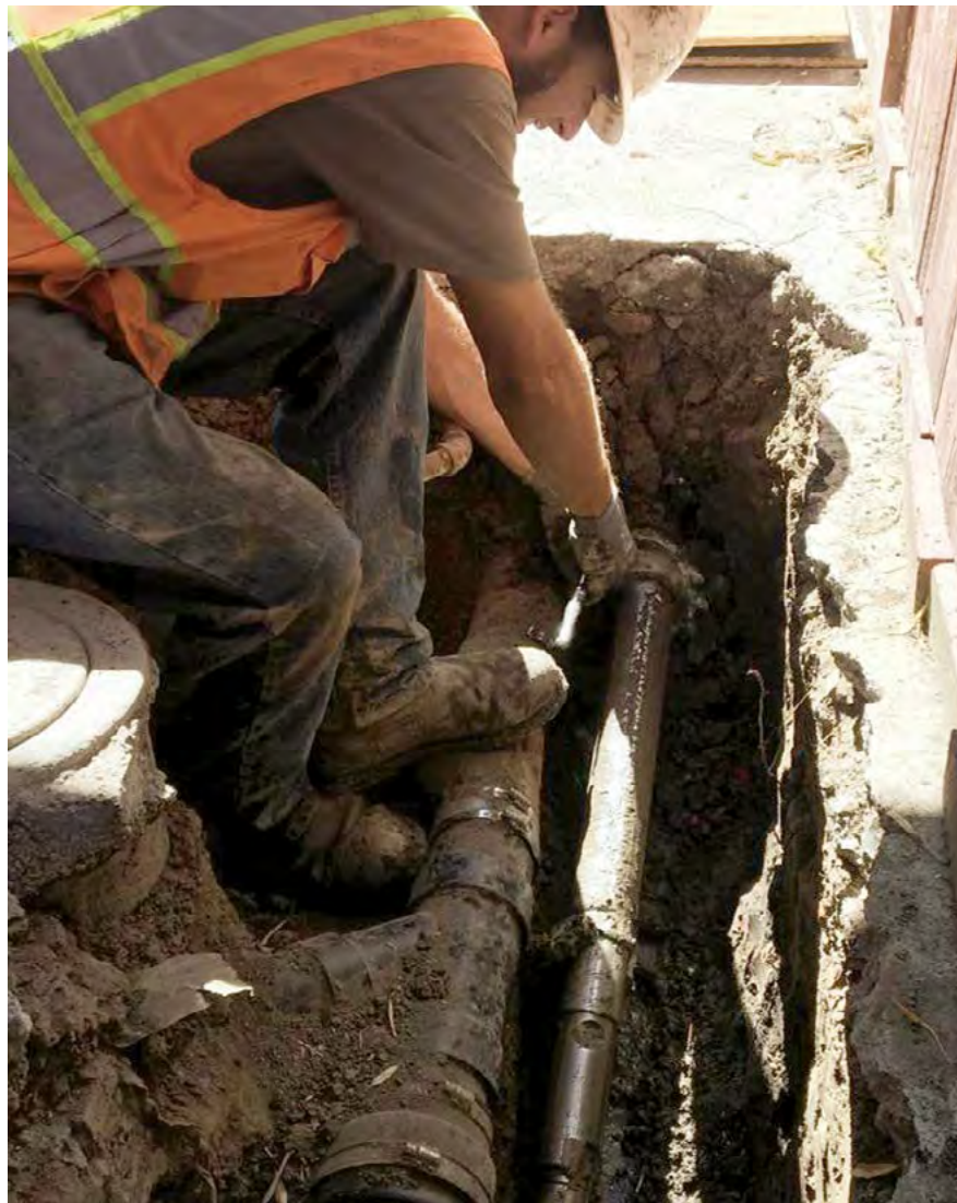
An example of the FastBack System boring close to existing utilities as well as in tight, closed-in conditions. In this instance it was a fiber installation next to a sewer main and a fence. The driller was able to pull his utilities without removing any structures or disrupting any existing utilities
