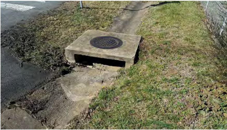
Maintaining aging infrastructure is a continuous challenge
