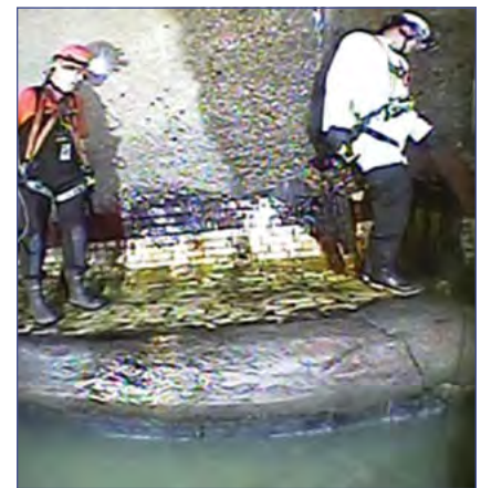
In this stretch of sewer, the walls show signs of moisture normally not seen in other sections, and much of the bench has failed and been repaired.
