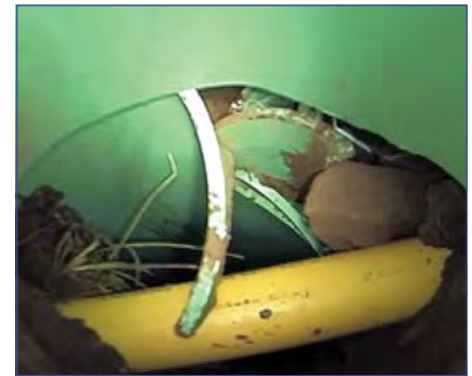
For a plumber hired to clear a clogged sewer line, a cross bore can be a catastrophic event.
