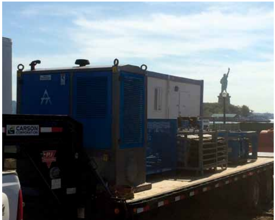
Static pipe bursting system, Quicklock bursting rods and the hydraulic power pack are on the trailer, ready to deploy, in the shadow of the Statue of Liberty
