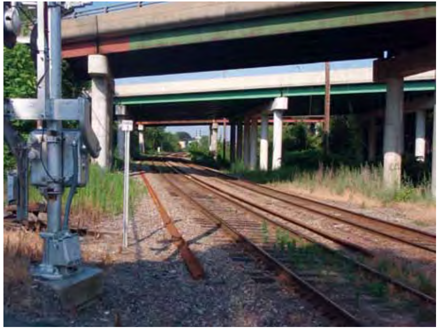
CIPP helped improve worker safety by allowing the pipe to be rehabilitated underneath the nearby railroad while commuter trains continued their regular schedule
