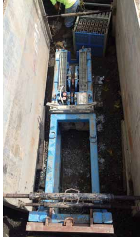
Carson Corporation used a Grundoburst 800G static pipe bursting system to burst and replace approx. 3,000 feet of 8-inch ductile iron water main with 10-inch HDPE
