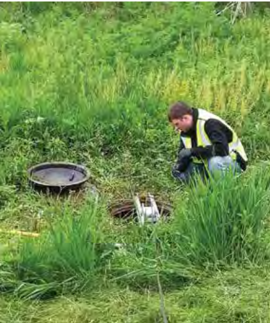
Pete Dannenberg of Electro Scan monitors the Electro Scan ES 620 probe as it is deployed through a manhole located in a low-lying wetland adjacent to Fern Creek
