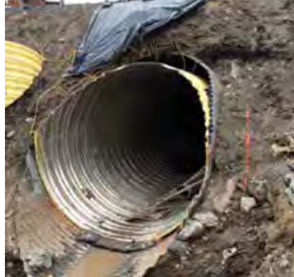
Lining the existing host pipe with tunnel liner plate provided the ability to build a safe working environment inside an unstable structure
