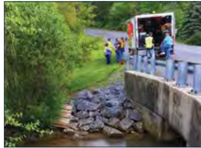
Figure 4: Scanning the PVC pipes adjacent to the creek, which was suspected to be the cause of the pipe infiltration.
