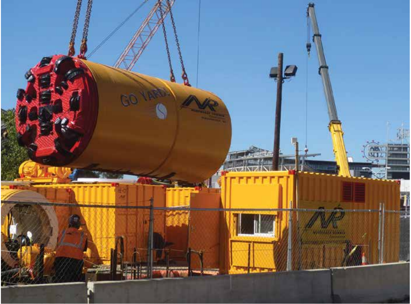
Launch shaft site on Tingey Street with Washington Nationals stadium in background
