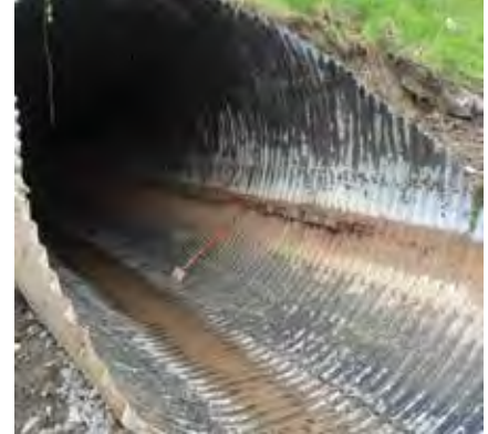
Two of the three original culverts had full depth corrosion along the entire length
